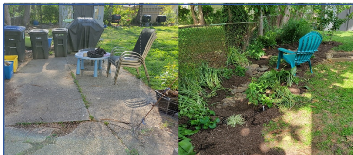
Pavement removal before (left) and after (right). Image credit: Chesapeake Bay Trust
