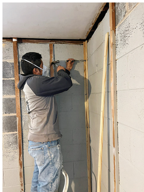
Village volunteer installs paneling after repairing a serious basement leak on Ritchie Avenue.
