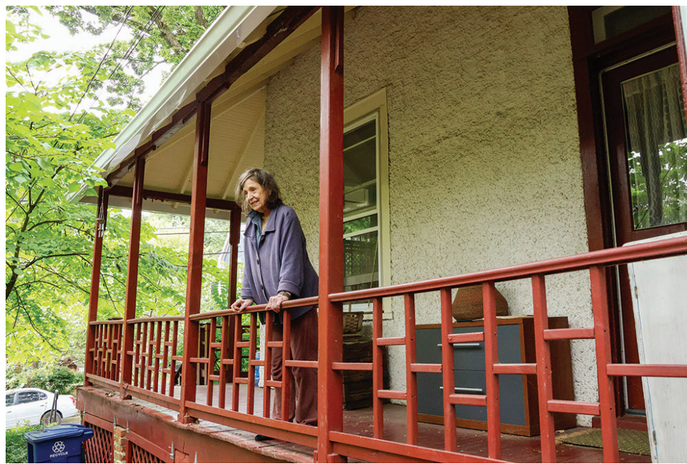
Village member Julie Boddy with new gutters installed to address interior water damage.
